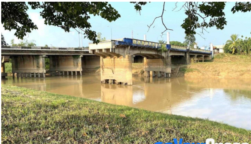
Jambatan putus buloh kasap broken bridge buloh kasap
